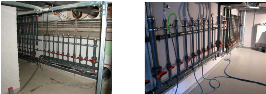
Figure 3 – Cooling water supply outlets. Left: the pump room, right: vacuum chamber hall
