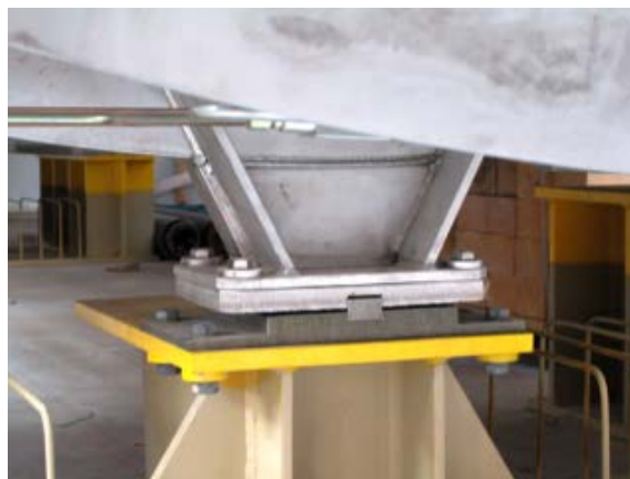
Figure 5 – View onto one of the sliding bearings on the vacuum chamber foundation
